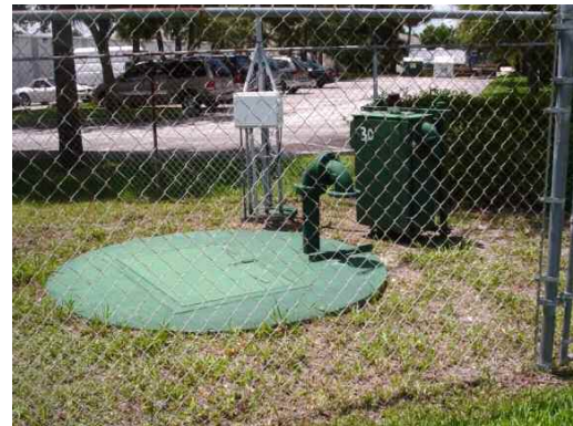
Lift Station Odor and Airborne Bacteria control
